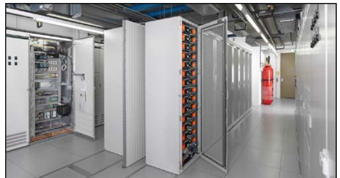
Figure 3: Battery energy storage system (BESS), Photo Siemens
