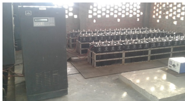
Figure 4. Solar inverter and batteries at Chakai plant
