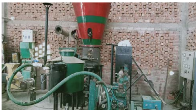
Figure 2. Biomass Gasifier Power Plant at Chakai village
