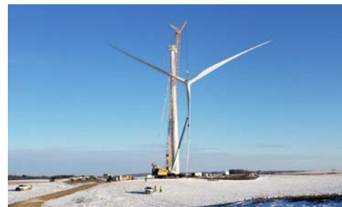
Fig. 6. The GE 2.0-116 rotor being lifted in place (Source: North American Wind Power)
