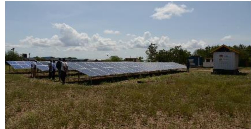
Standalone solar system with containerised battery bank
