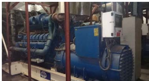
Figure 2. F.G. Wilson heavy oil generators
