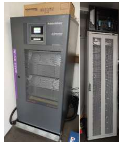
Figure 8 Socomec NMC ESS (converter on the left, battery on the right)
