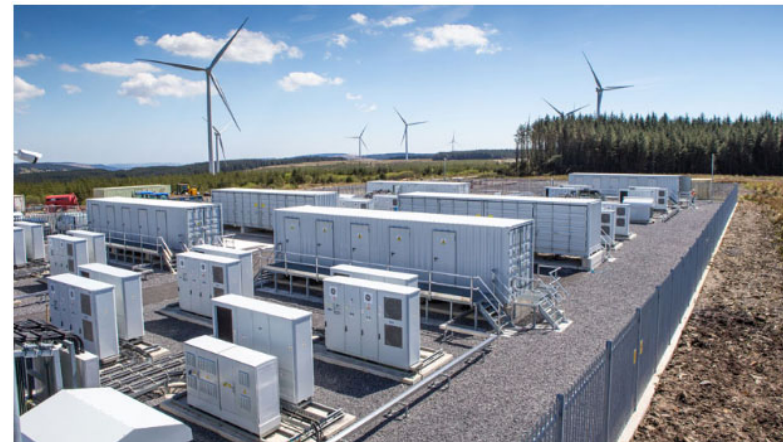
Battery storage at the Pen y Cymoedd Wind Farm in the UK, source: Vattenfall
