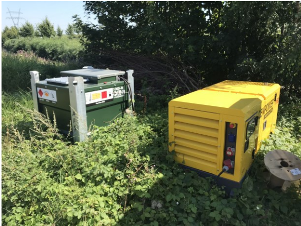
Diesel genset incl. fuel supply on site, 30 kVA
