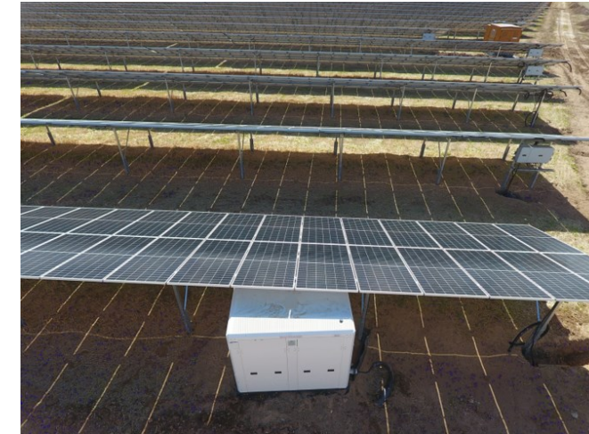
mobile battery below PV tables with DC connection of strings
