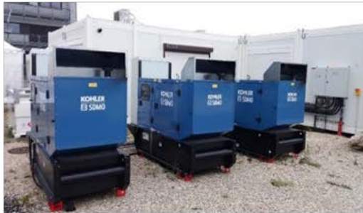
Diesel Generators (3* 44 kVA)
