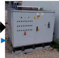
Load bench (125 kVA)
