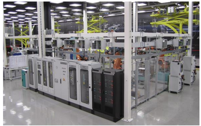
Figure 4 DC microgrid realization as automotive manufacturing cell for experimental analysis.
